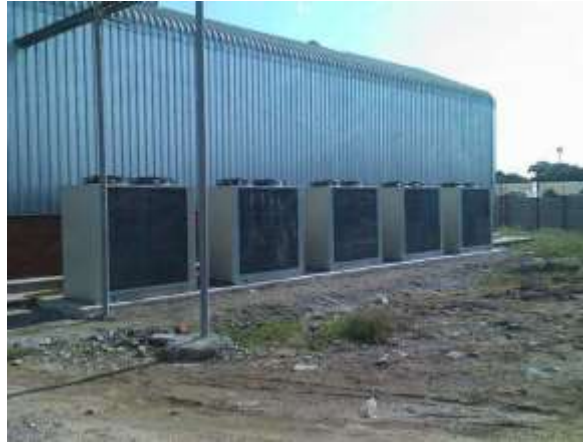
Figure 2: Photo of a heat pump installation.
